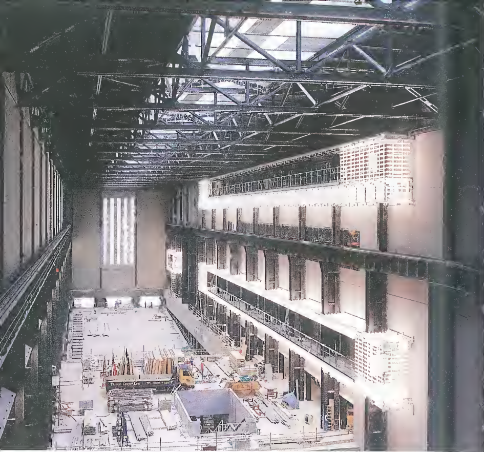
The turbine hall of Bankside Power Station during conversion into Tate Modern.
